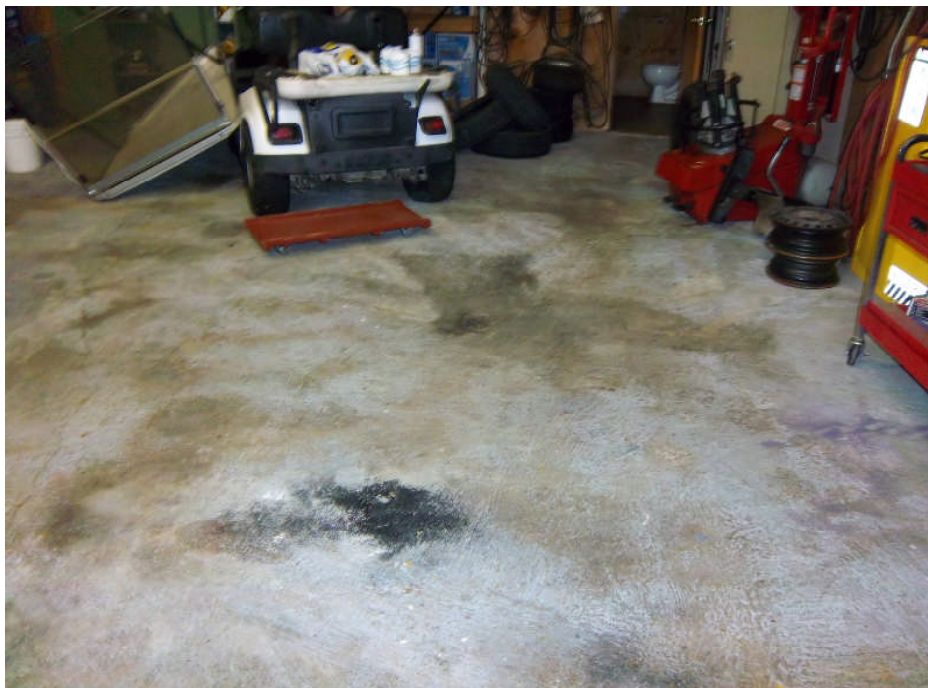
Photograph 18: View of the interior of the vehicle maintenance shop looking north at the floor drain and dark staining on the concrete floor.
