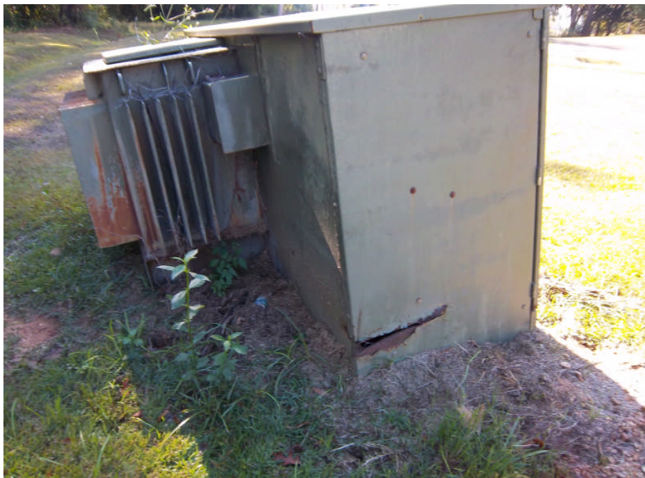
Photograph 20: View of the north side of the electrical transformer showing the gash in the housing approximately 4-5 inches above the ground surface.
