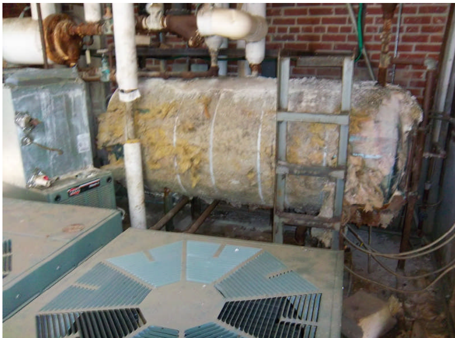
Photograph 12: Typical view of the interior of the cafeteria boiler room.
