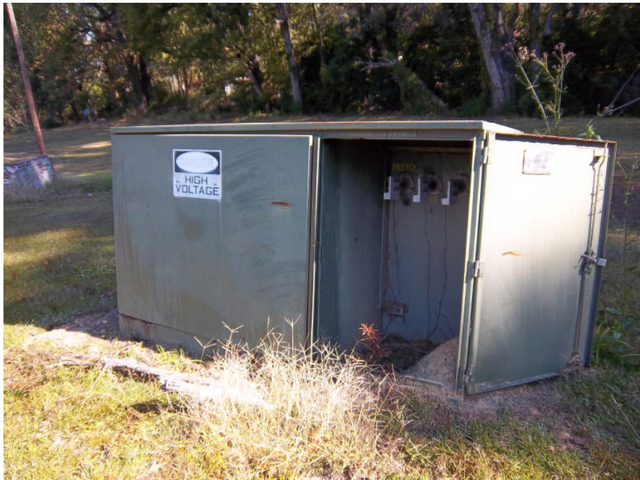
Photograph 19: View of the electrical transformer housing stored on the ground surface east of the used oil AST.
