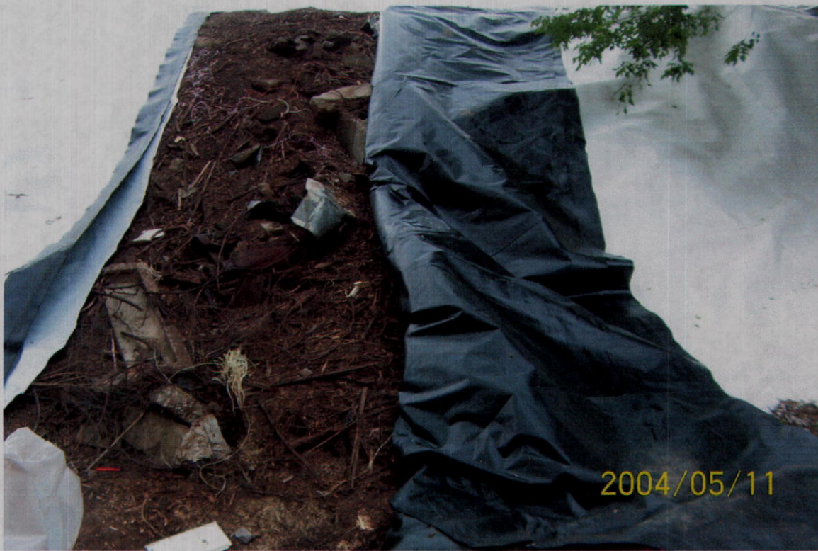
PHOTO 11 – A view of Test Pit #2 on the west side of the fill area prior to excavation. Test pits were placed in areas containing significant quantities of metallic and non-metallic debris. Photo was taken from the toe of the slope.
