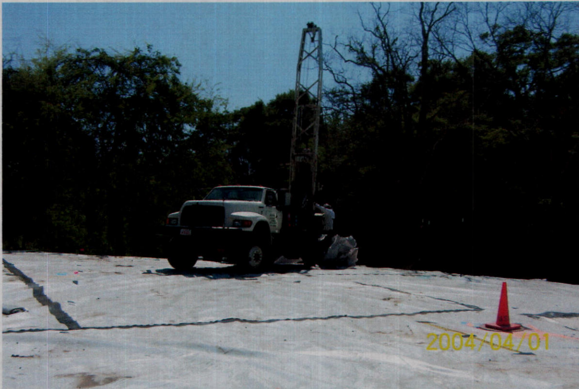
PHOTO 7 – Drillers positioning hollow stem auger drill rig on the western slope of the fill material on the 114 Brent Street MSL property.
