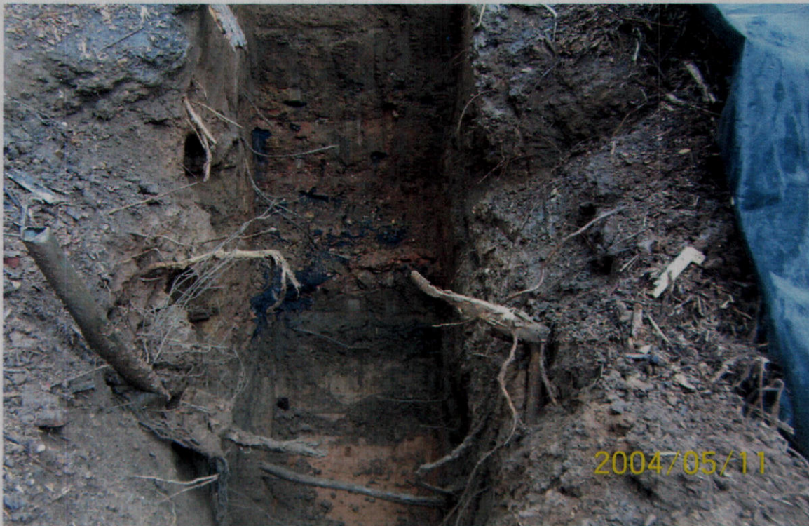
PHOTO 17 – A view of a completed test pit. Note transition zone between fill material and native red, sandy soils at the bottom of the pit.
