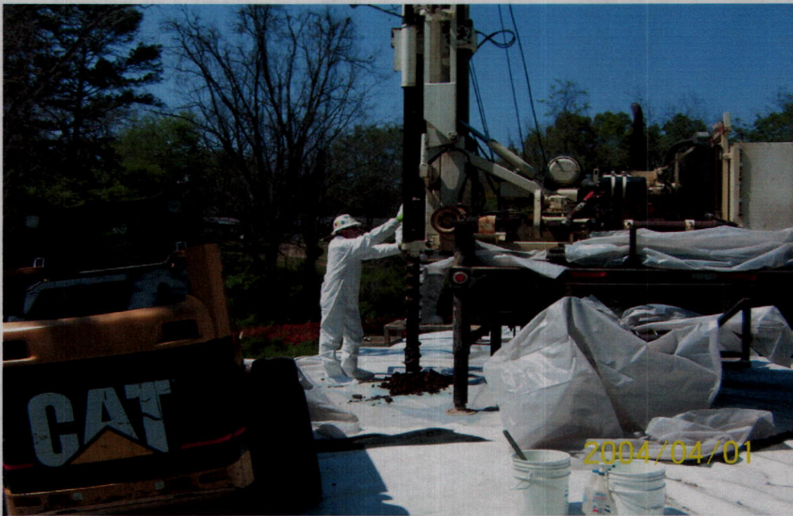
PHOTO 8 – Installation of hollow stem auger boring on the western slope of the fill area at 114 Brent Street. Boring locations were selected based on results of the geophysical survey and were placed in areas identified as containing minimal quantities of subsurface debris.
