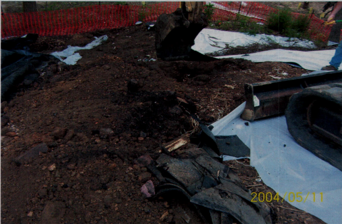
PHOTO 18 – A view of Test Pit #4 from the top of the southern slope after backfilling. After backfilling activities were completed, the HDPE liner was placed back over the excavated area and thermally sealed.
