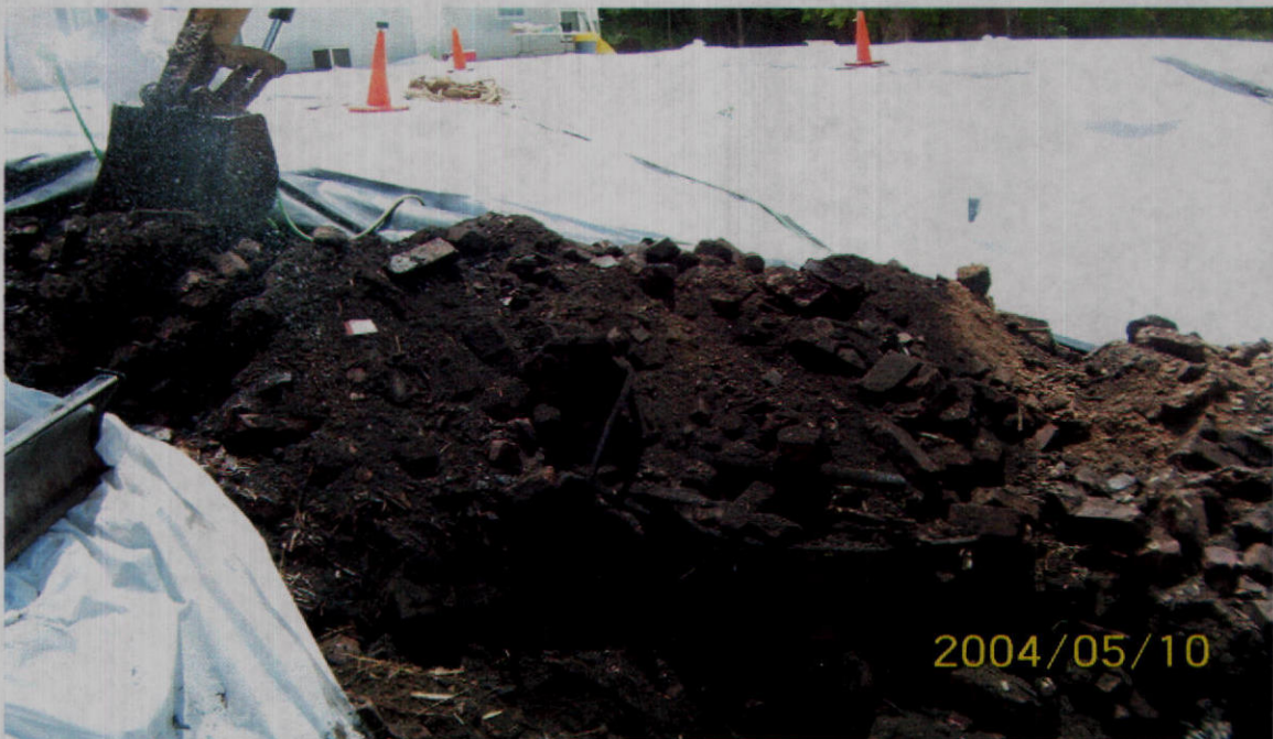
PHOTO 14 – View of the stockpile of typical metallic and non-metallic debris encountered during this phase of the assessment. This material was excavated from Test Pit #5 on the southeastern slope of the fill area. Photo was taken prior to backfilling the test pit.
