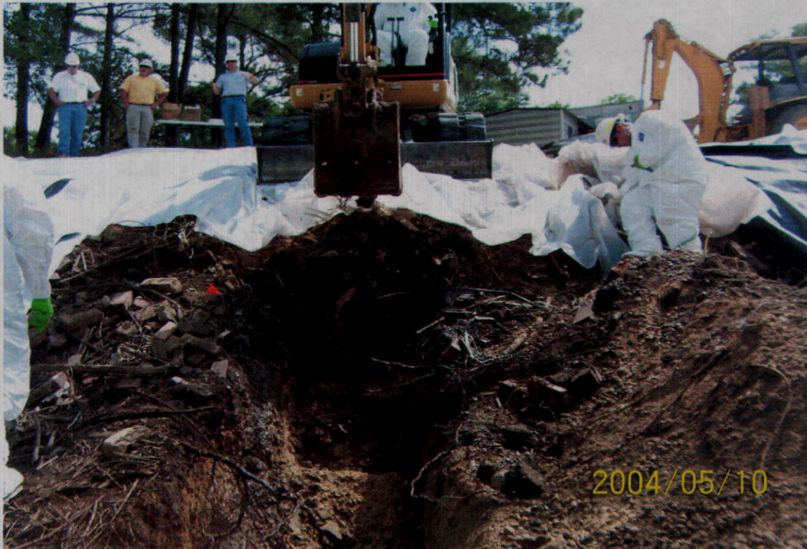
PHOTO 13 – Excavation of Test Pit #2 on the northwestern slope of the fill area. Photo was taken at the toe of the slope looking west to east.
