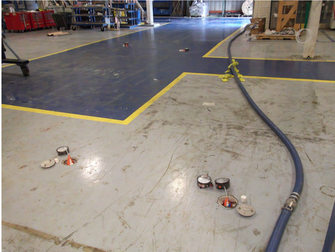
Monitoring Vacuum at Observation Wells 20 feet from extraction well
