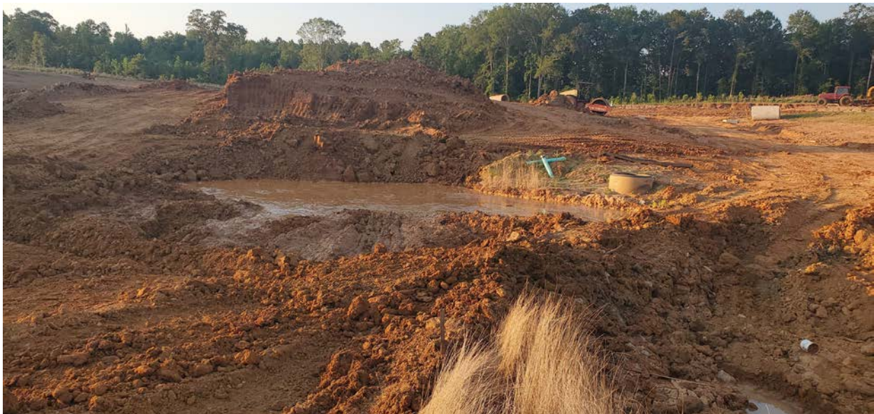
Figure 3-1. Soil exposed during construction is subject to erosion and may contribute to NPS pollution if sites are not properly managed. (Photo: Natalie Segrest, MDEQ)
