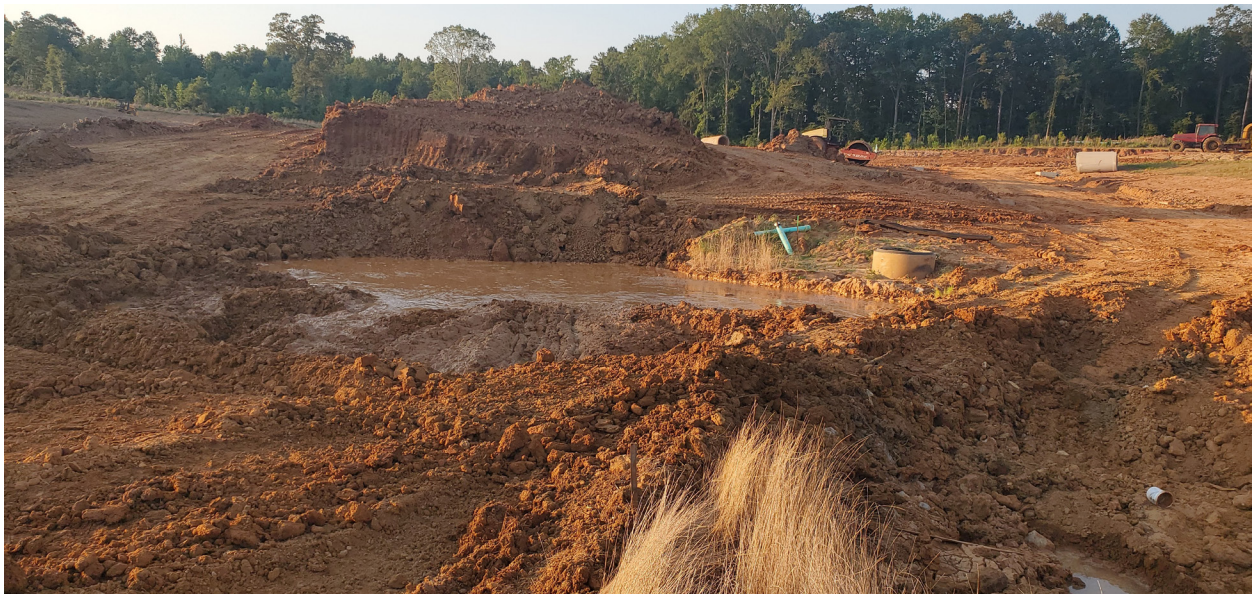
Figure 3-1. Soil exposed during construction is subject to erosion and may contribute to NPS pollution if sites are not properly managed. (Photo: Natalie Segrest, MDEQ)
