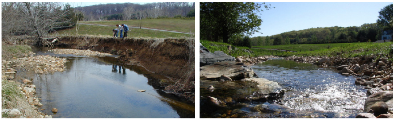
Figure 2-21. Minebank Run in Baltimore, MD. Before (left) and after (right) stream restoration. (Source: USEPA Archives)
