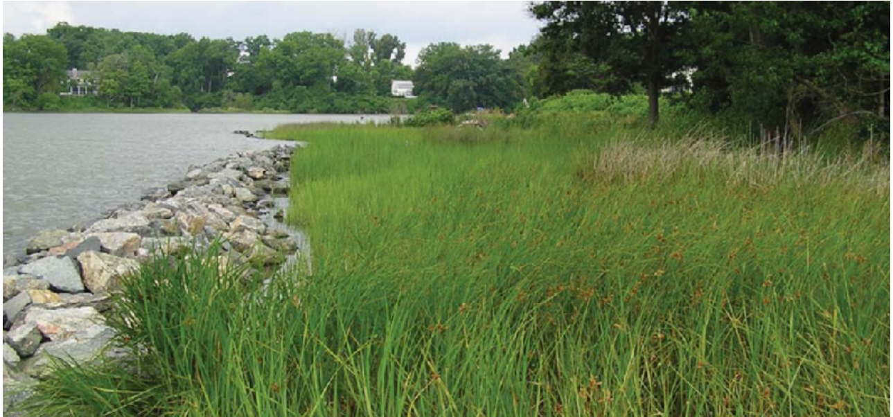
Figure 2-22. Rock sill with planted marsh, an example of hybrid design employing structural stabilization and living shoreline techniques. (Photo: K. Duhring, MDMR)
