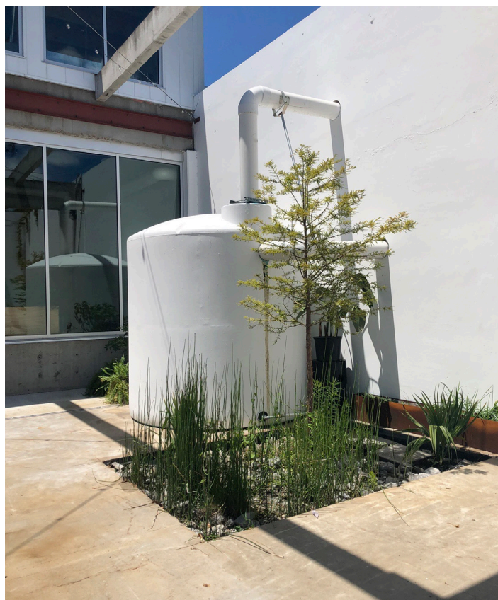
Figure 2-17. Rooftop downspouts directed to cistern and stormwater planter at Ecoshed in Jackson, Mississippi.
