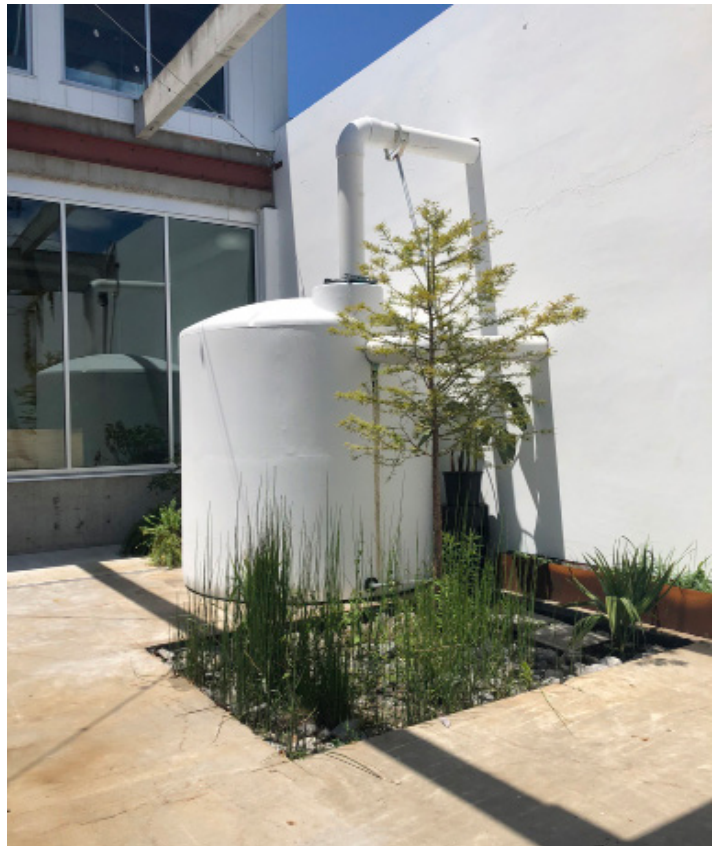
Figure 2-17. Rooftop downspouts directed to cistern and stormwater planter at Ecoshed in Jackson, Mississippi.
