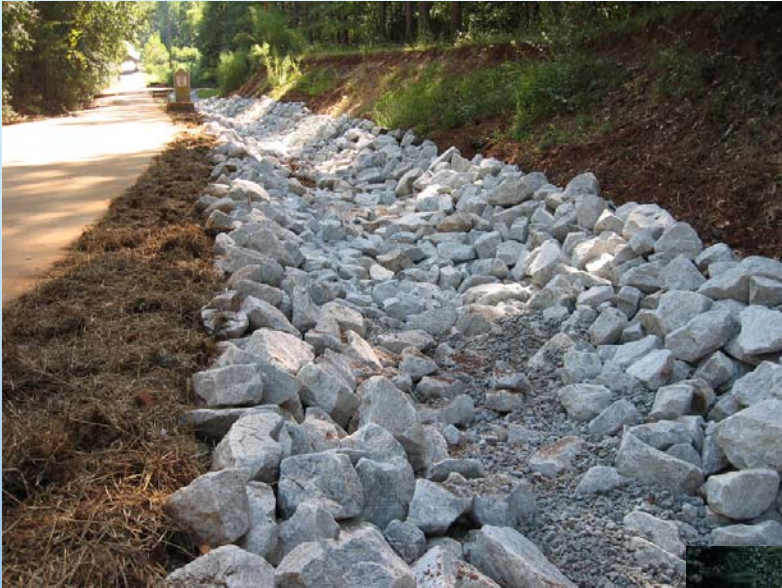
Granite Rip Rap Rock Drainage Swale
