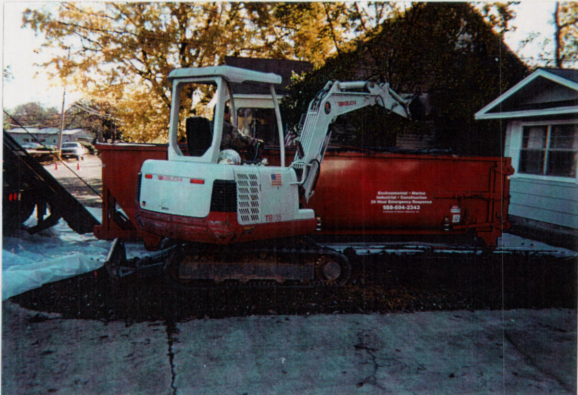
Newman Duplex property looking east showing excavation of the median strip between the two driveways.
