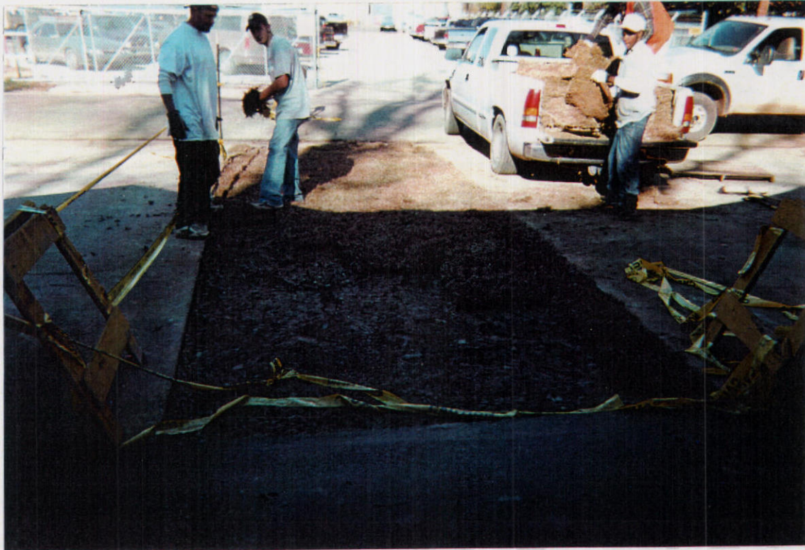
Newman Duplex property looking north showing new sod being installed on the clean backfill.
