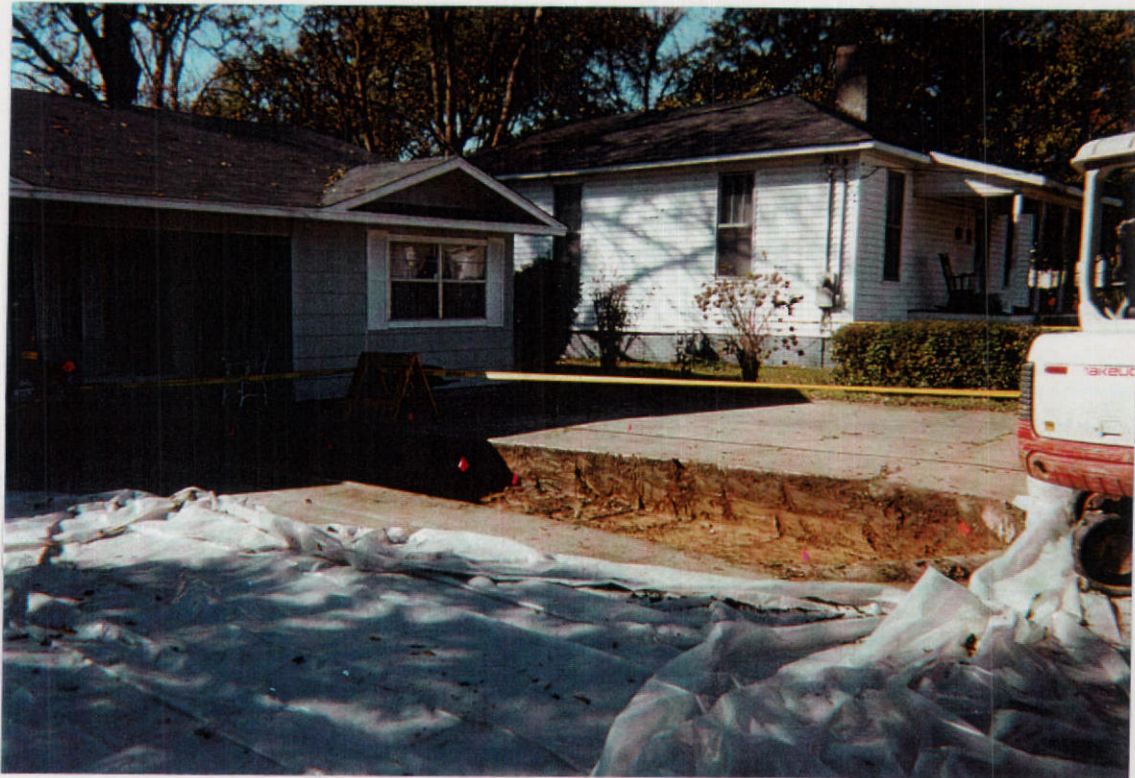
Newman Duplex property looking southwest showing the completed excavation with sample locations marked by red flags.
