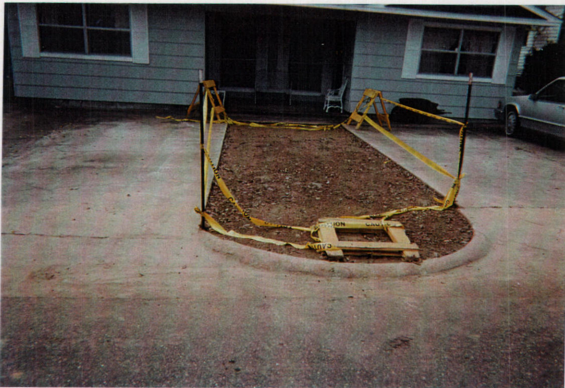
Newman Duplex property looking south showing the excavation filled with clean soil following confirmation that all contaminated soil was removed.
