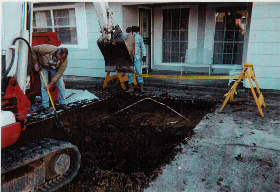
Newman Duplex property looking southeast showing excavation of the median strip between the two driveways.
