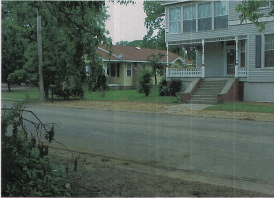
Photo 7 – Completed excavation along Lee Avenue with backfill in-place. View is looking northwest across Lee Avenue.
