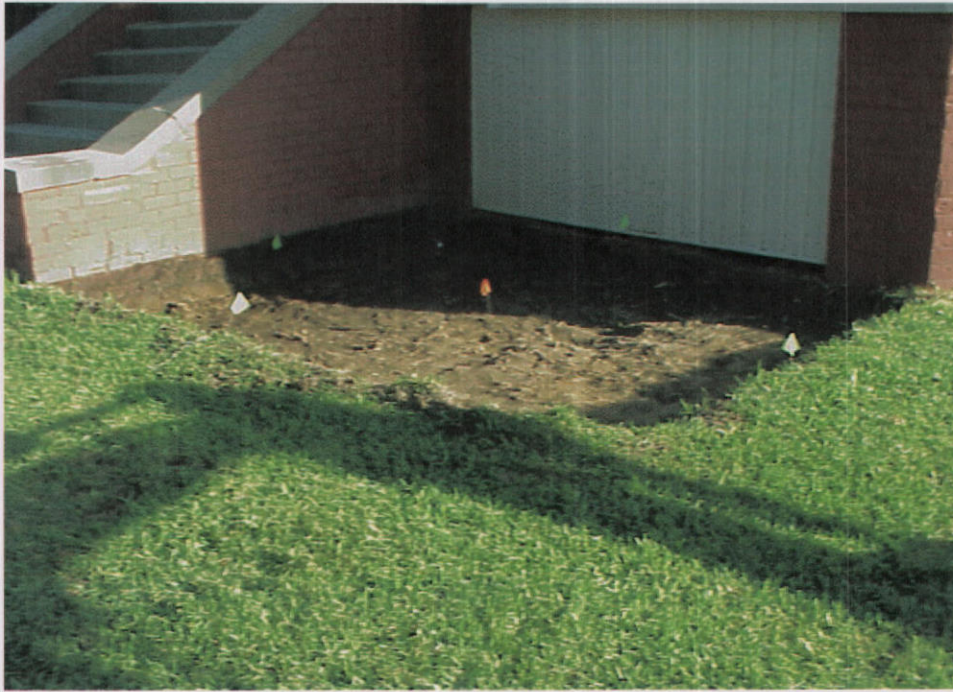
Photo 5 – Completed excavation on the northeast side of the Frazier's front porch. Flags marking confirmation sampling locations are visible in the excavation.
