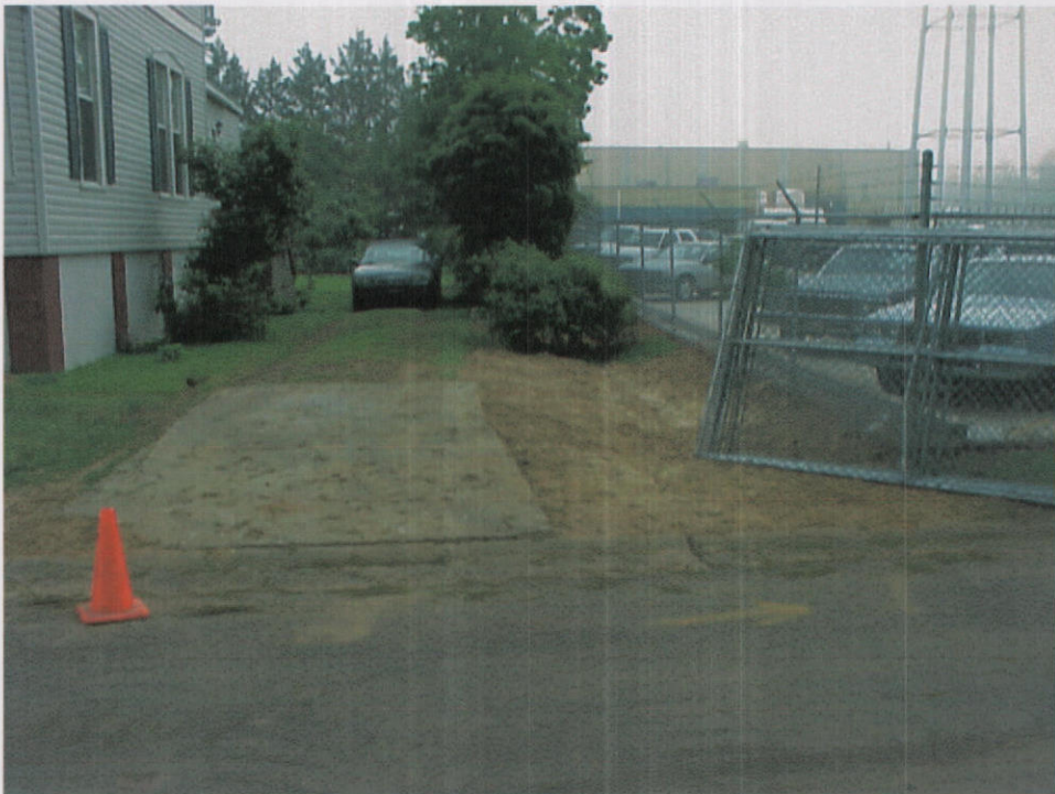
Photo 8 – Completed excavation between the driveway and Kuhlman Electric's parking lot with clean backfill in-place and graded. This view is toward the north across Lee Avenue.
