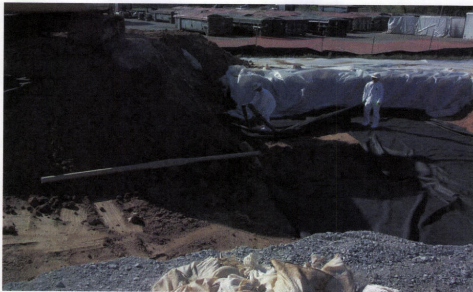
PHOTO 12 – Geotextile fabric being installed at the base of a deep excavation at the northeast corner of the plant building.
