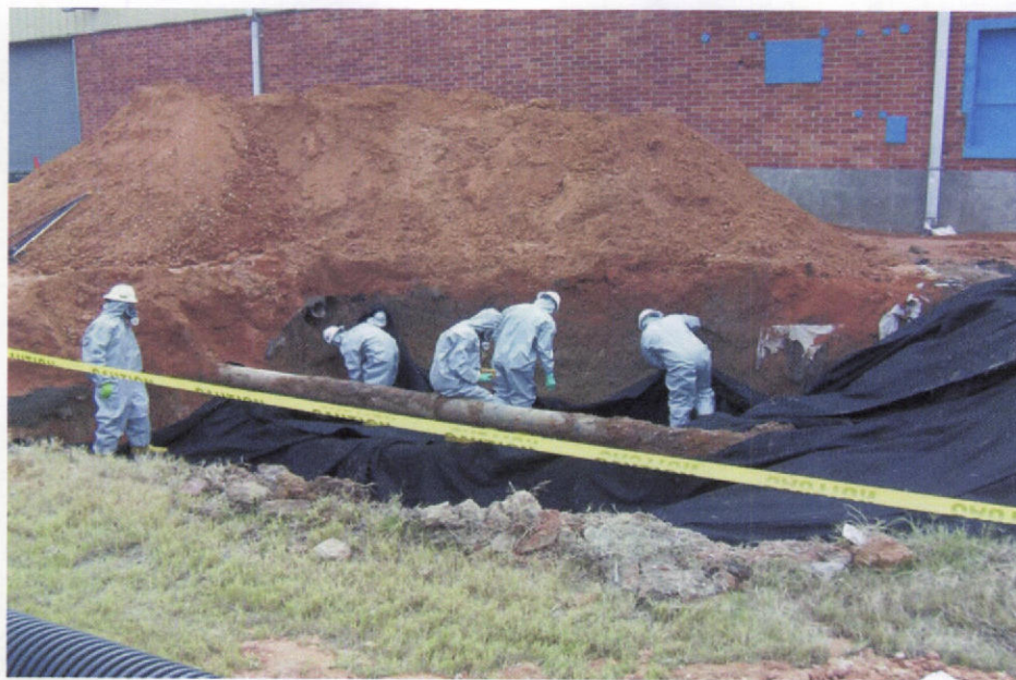
PHOTO 20 – View of the same excavation as the previous photo looking southwest. The stockpile of soil in the background is clean backfill staged for use in the excavation.
