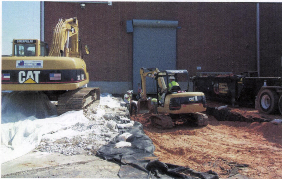
PHOTO 10 – Location of this view is at the northeast corner of the plant building looking south. Backfill is being placed in the excavation over geotextile with the aid of a small excavator.
