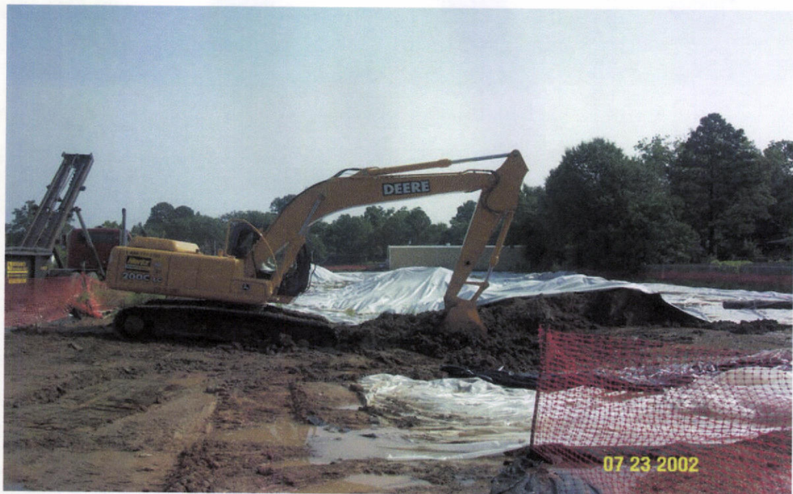
PHOTO 6 - Photo taken looking north on east side of the plant property showing removal of Stockpile #1. Also shows the limited uncovered working area.
