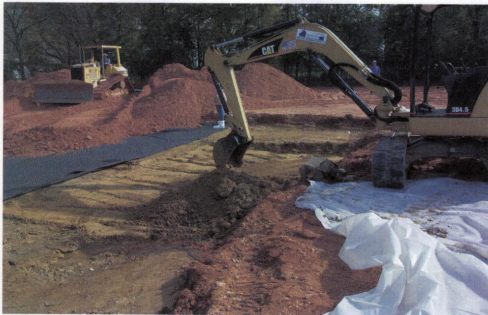
PHOTO 8 - View of the excavation activities. The dark geotextile fabric underlayment is visible in the left background. Clean fill soil is being graded over the geotextile.
