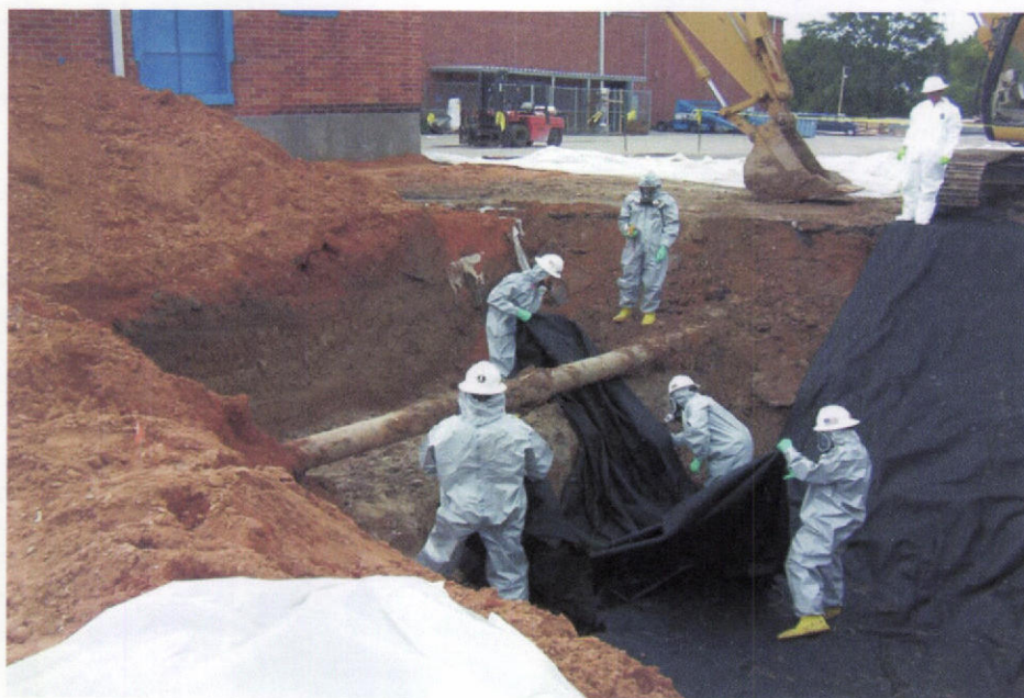
PHOTO 19 – Workers spreading geotextile in a deep excavation on the east side of the plant site. View is from the field on the east side of the plant looking northeast.
