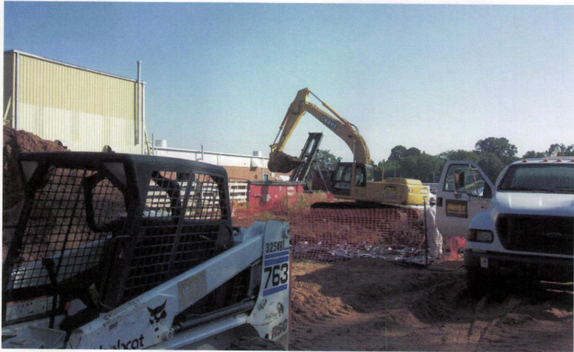
PHOTO 5 - Photo taken looking north on east side of the plant property showing soil removal activities.
