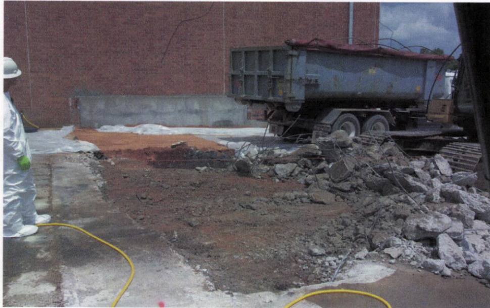
PHOTO 9 – Location of this view is at the northeast corner of the plant building. Concrete debris is being loaded into roll-off boxes for disposal. Worker at the right is providing dust control with a water spray.
