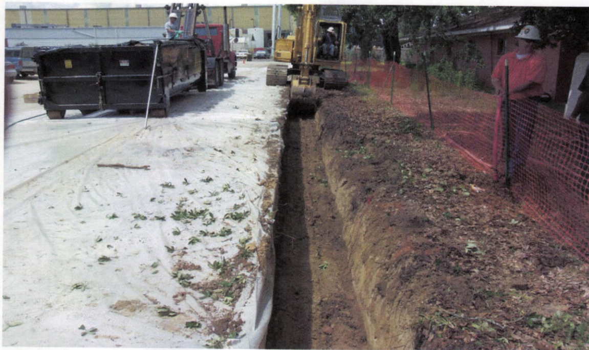
PHOTO 1 – Cutoff trench being excavated along the KEC property line common with the Medical Center property. Photo is taken looking north from Lee Avenue.
