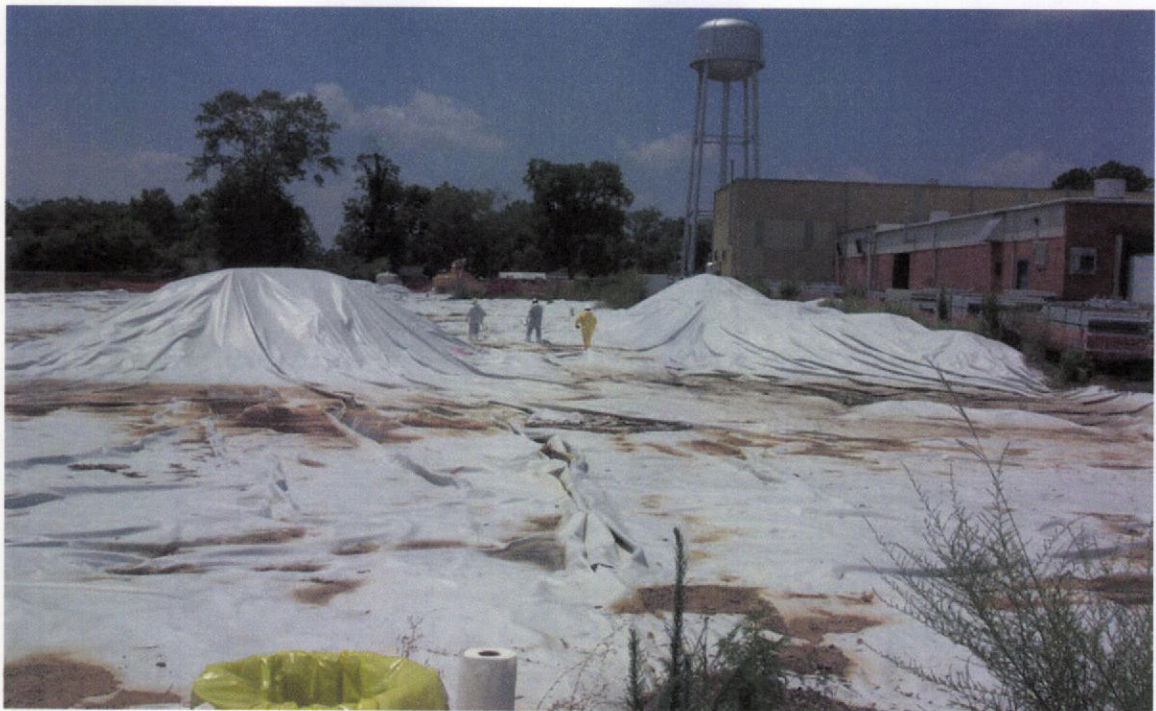
PHOTO 4 – View of the exclusion zone looking south showing the 12-mil HDPE liner coving the site. Photo taken prior to start of remediation activities.
