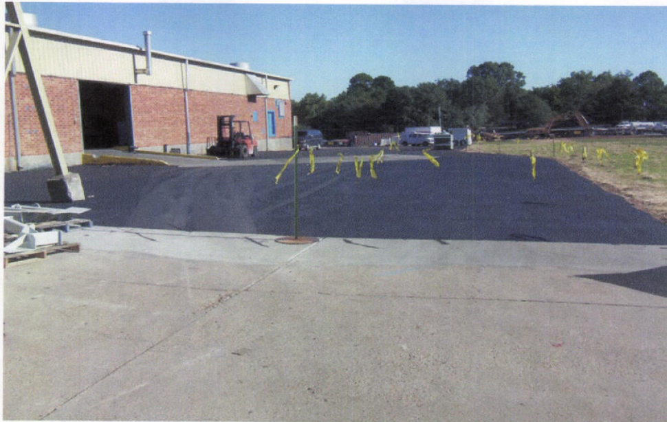
PHOTO 16 – View of the same area as the previous photo looking north along the east side of the plant building with the finished asphalt surface in place.
