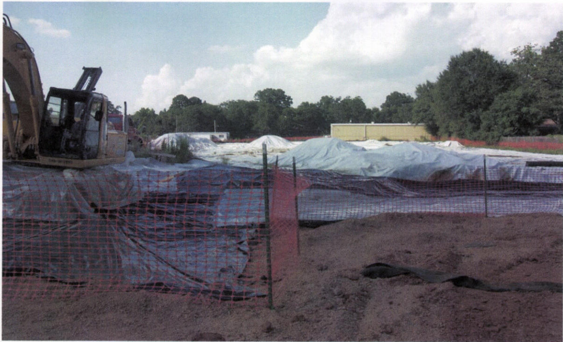
PHOTO 3 – Exclusion zone with temporary plastic cover installed at the end of the workday. The 12-mil HDPE liner is visible in the background. Photo taken looking north on east side of the plant property.
