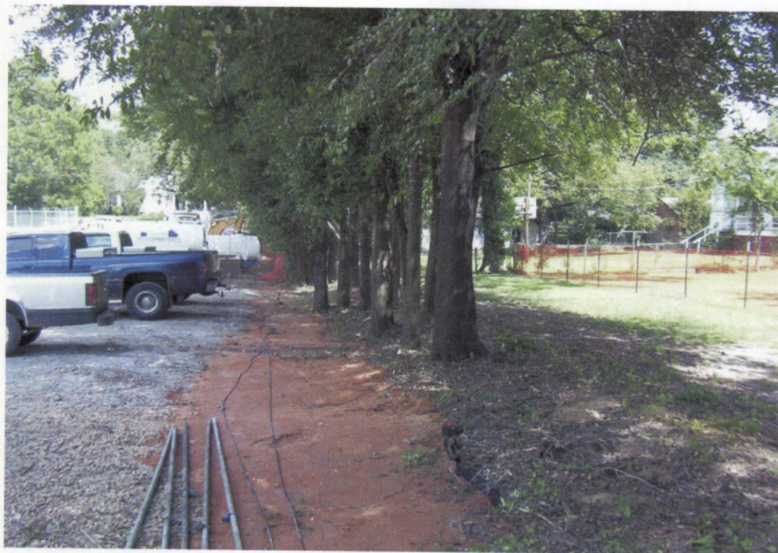
PHOTO 2 – Cutoff trench located along the east property line backfilled with clean soil.
