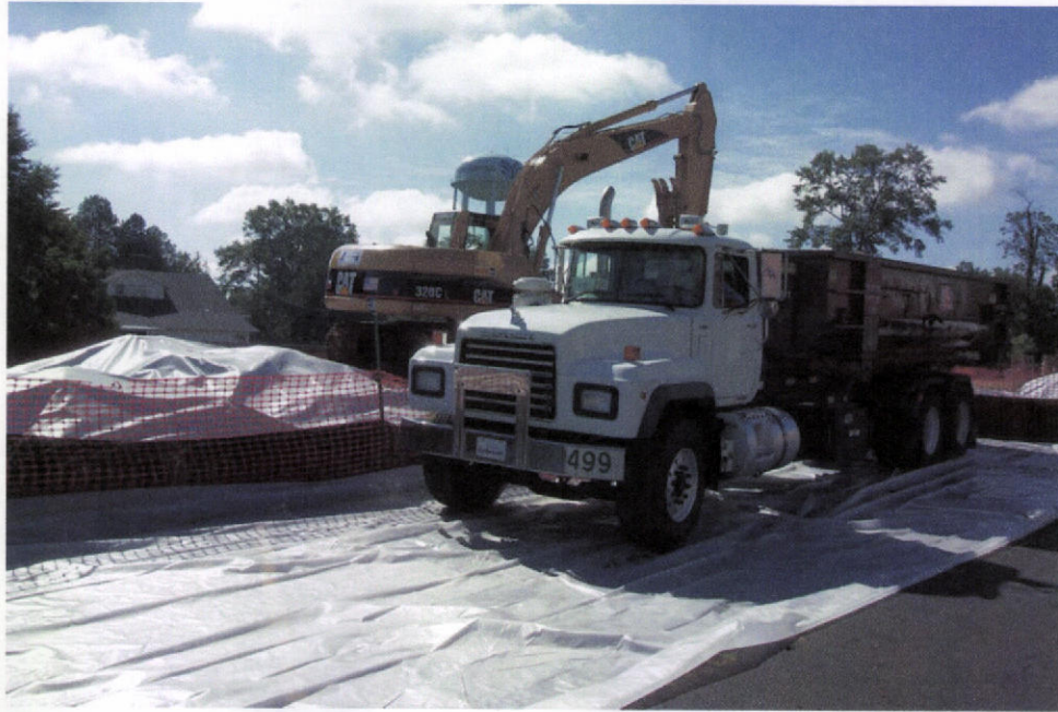
PHOTO 7 - The excavator is working in the exclusion zone loading impacted soil into a roll-off box parked on plastic outside the exclusion zone.
